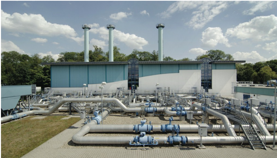
Figure: Compressor station operated by GVS (Reference: ENBW)
